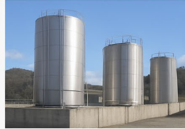
Product storage tanks
